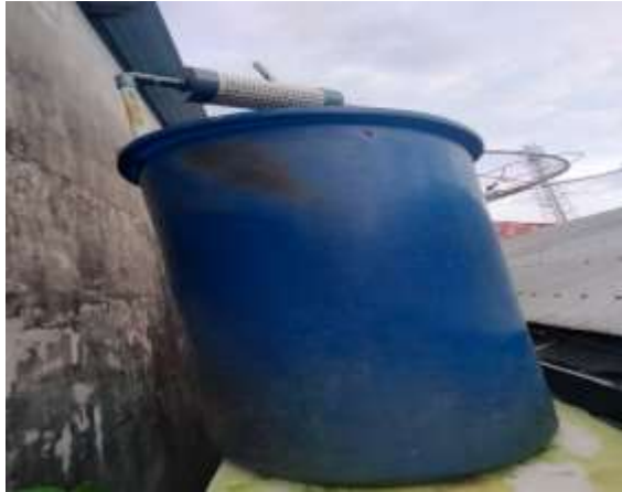
Pic 2. Aeration unit (aerator and reservoir)
